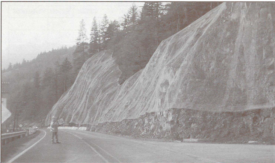
Route 14, Washington, north of the Little White Salmon River. The fencing on the cliff walls prevents rocks from falling onto the roadway. The Washington State Department of Transportation has assured us that they will be painting this fencing to make it less noticeable. The Friends is a key player in the planning process for the future of this scenic Gorge highway.
